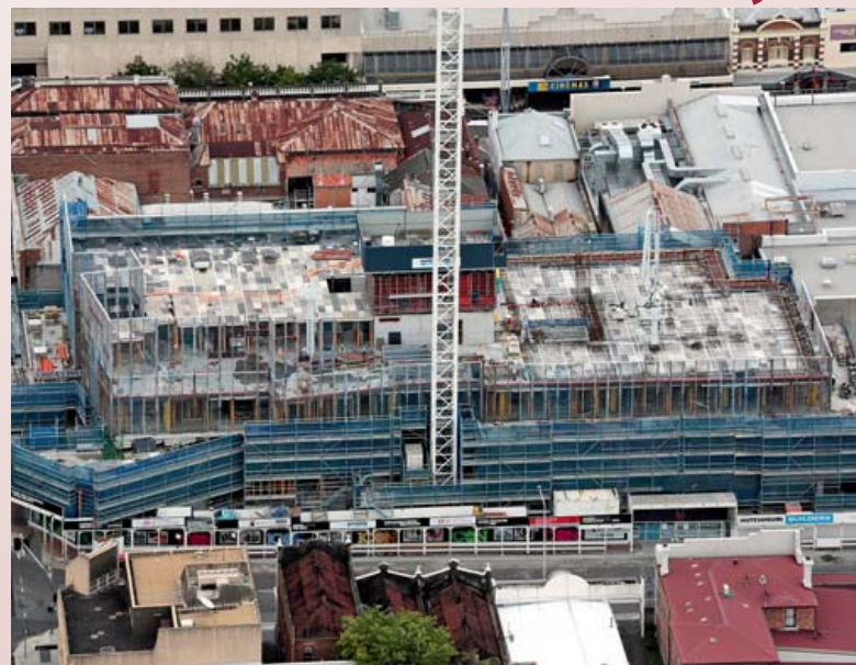
The beginning of a nine-storey tower in an urban renewal project in Ipswich's CBD.
